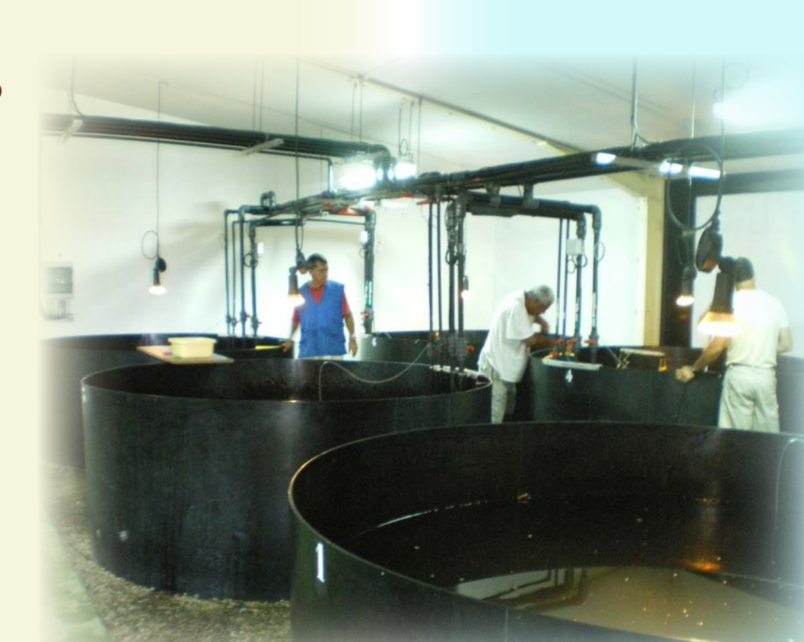
Picture 6 : maturation circular tanks
